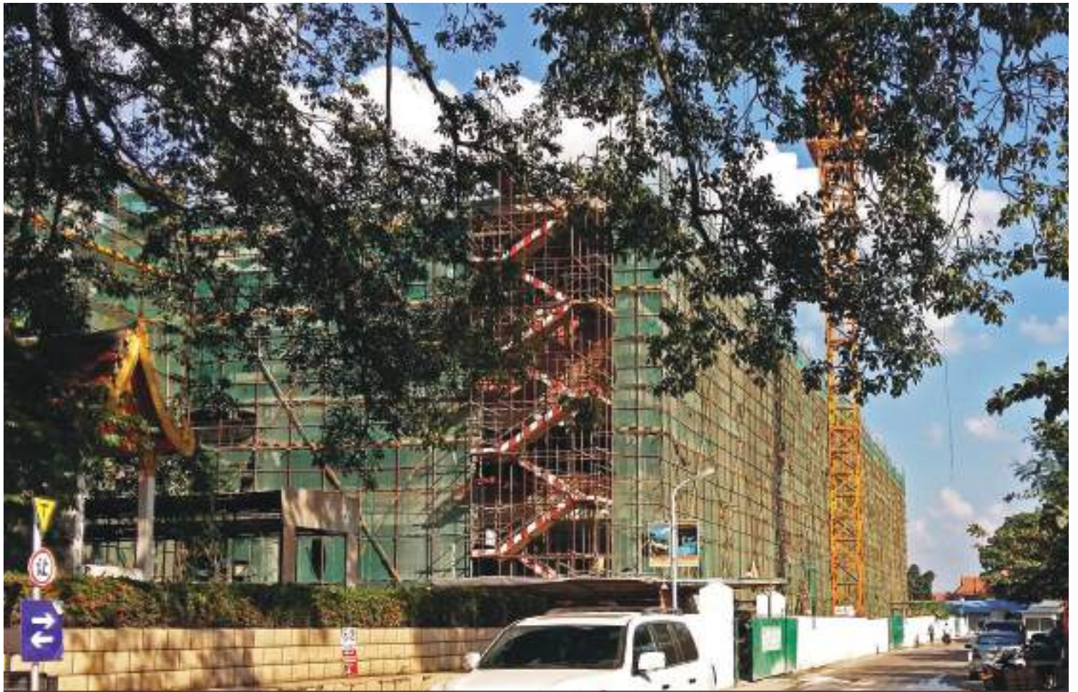
In 2015 scaffolding covered a large extension to Vientiane's San Jiang Chinese market, where many outlets selling recently-made ivory items can be found. The building was near to completion by late 2016.
